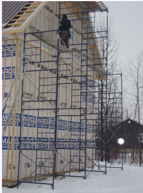
This scaffold has inadequate planking, missing braces no guardrails and should be tied into the structure
